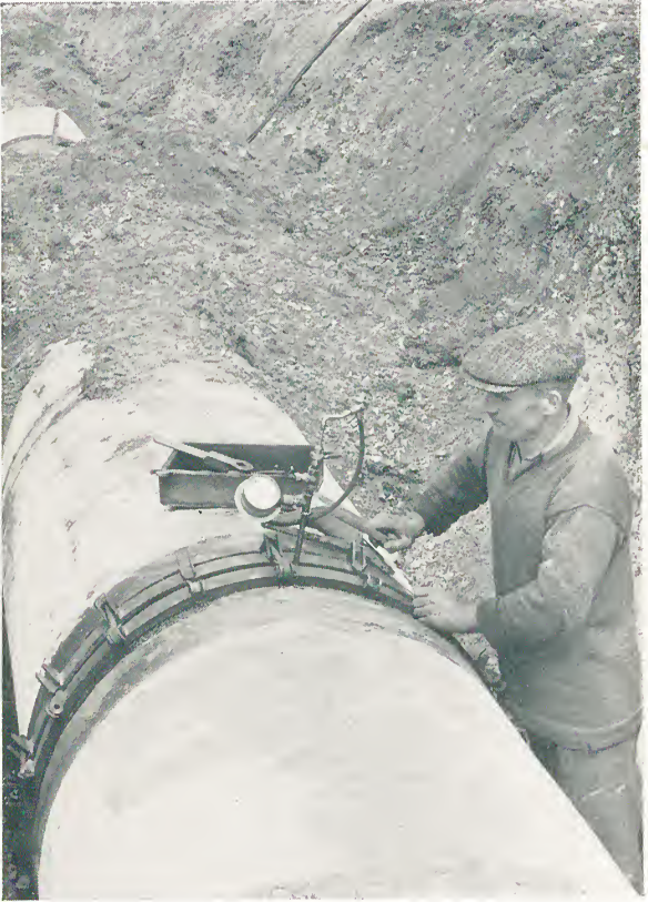
Testing an internally welded sleeve joint on an 'S & L' steel water main.
